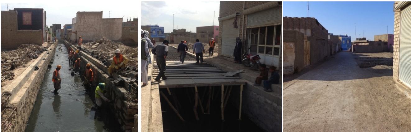
Municipal level project: The 1.3Km municipal infrastructure canal in Herat under construction (left and middle) and completed (Right). This project benefits thousands of men, women and children by reducing seasonal flooding risks and ensuring improved drainage for a large part of the city.
